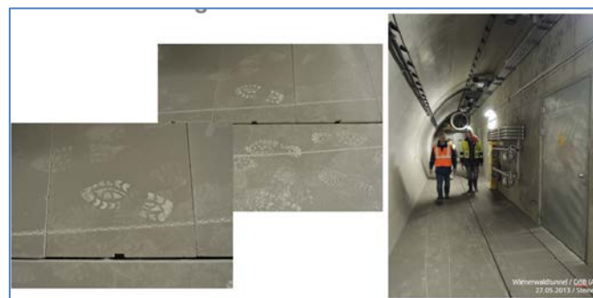
Figure 3: Dust load in a cross passage of the Wienerwald Railway Tunnel / ÖBB Westline
